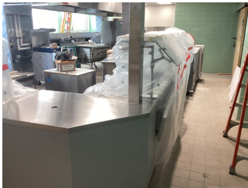
Kitchen Equipment Installed
