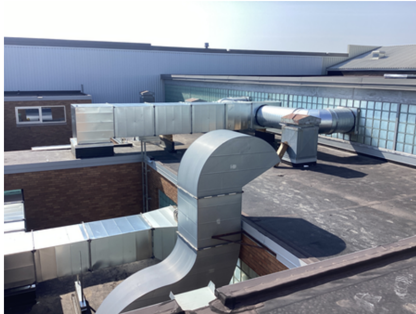
Ductwork and mechanical equipment for competition gym
