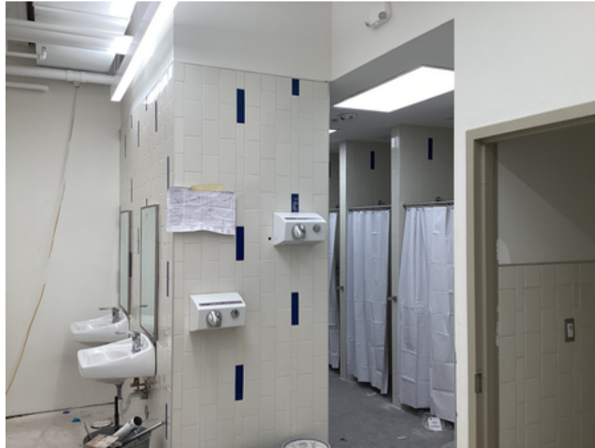
Plumbing fixtures and finishes in boys locker room
