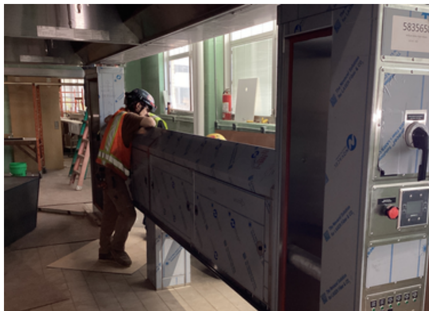
Kitchen equipment mechanical/electrical distribution
