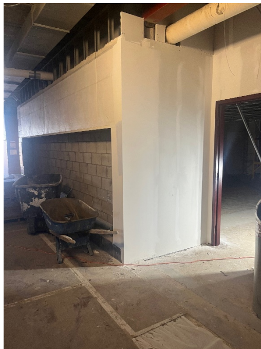
Locker Bases and Soffits
