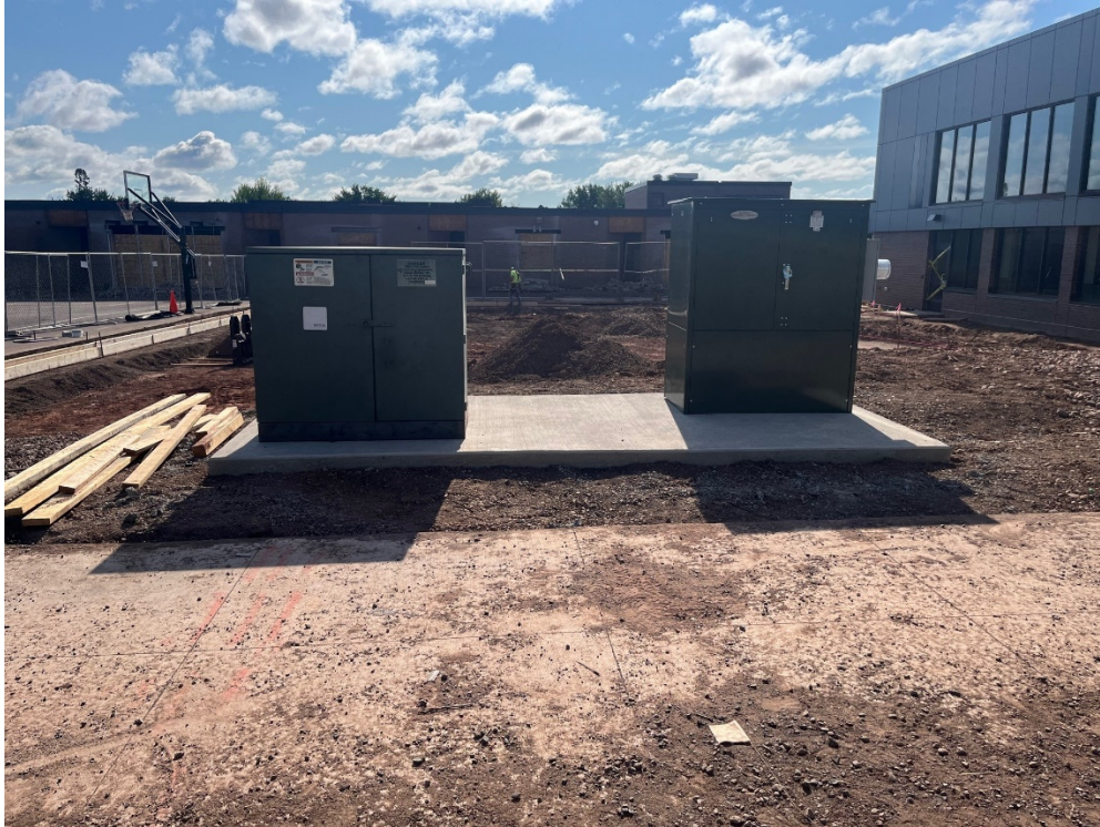
New Transformer Set.
